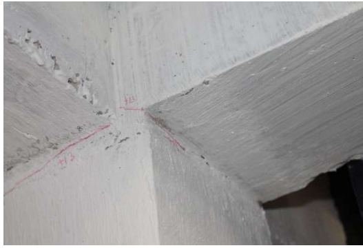
(a) First flexural crack in the column
