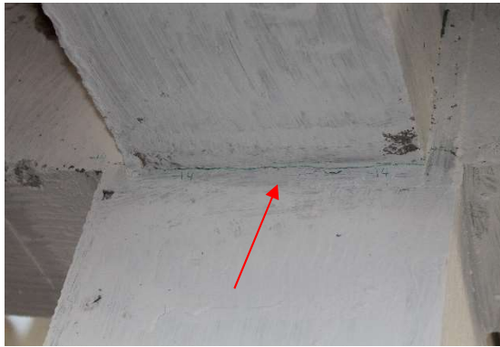
(a) First flexural crack in the columns
