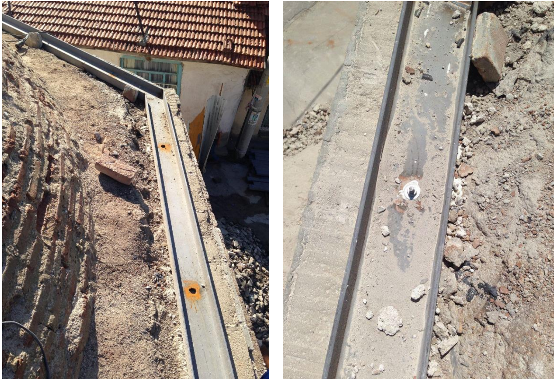
Figure 2.18. Single bar U160 steel girder at the top section of the drum and anchorage connection
