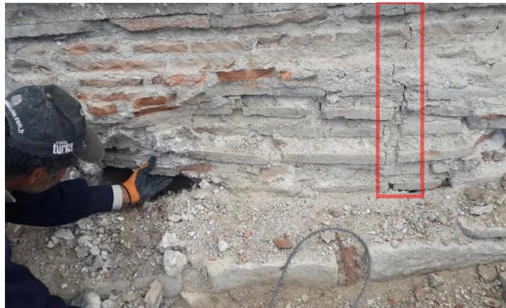
(a) Exterior crack on the octagonal drum
