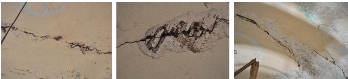
(b) Crack observed on the intrados
