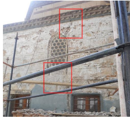
(b) Cracks on the east façade
