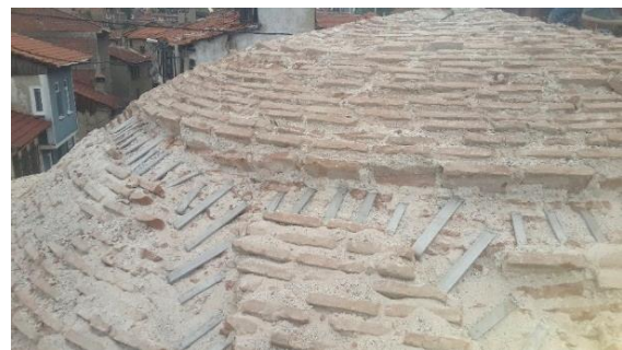
(b) Stainless steel elements along the crack
