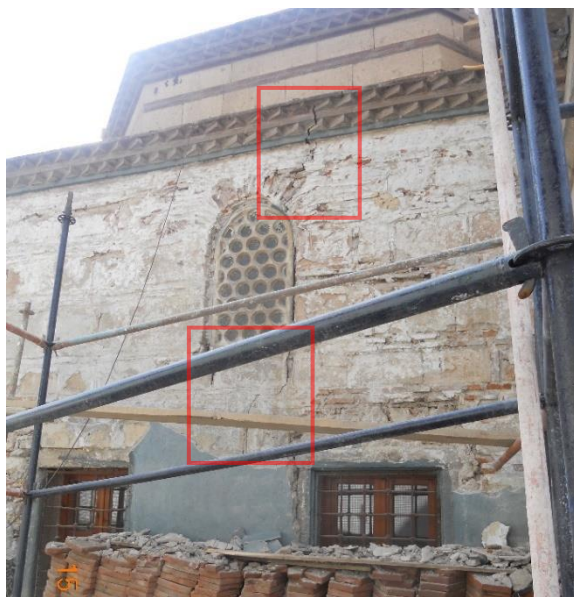
(a) Vertical crack on the East façade
