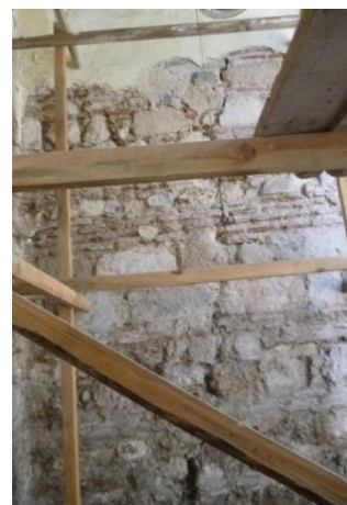
(b) Crack on the West Portico Wall, inner layer
