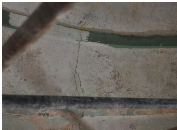
(b) Interior crack on the octagonal drum
