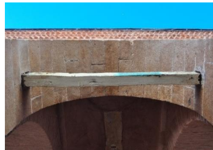
(b) Material decay on the wooden tie beam
