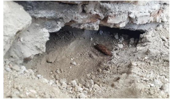
(b) Loss of wooden beam
