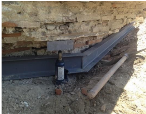
(a) Steel girder at the bottom section of the drum
