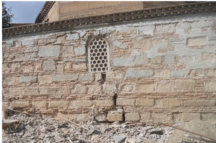
(a) Vertical cracks
